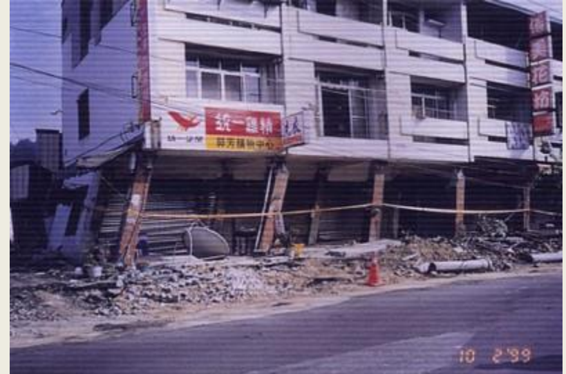
Chi Chi 1999 Taiwan earthquake
